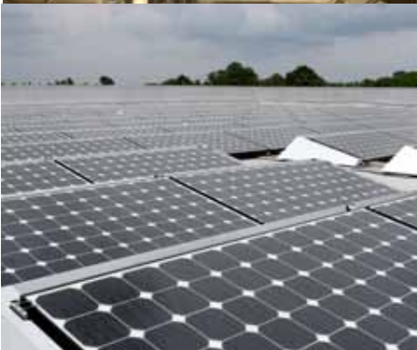
TOP: The NIH Library's green features include a green terrace with plants and solar panels. (Photo by Bradley Otterson)
